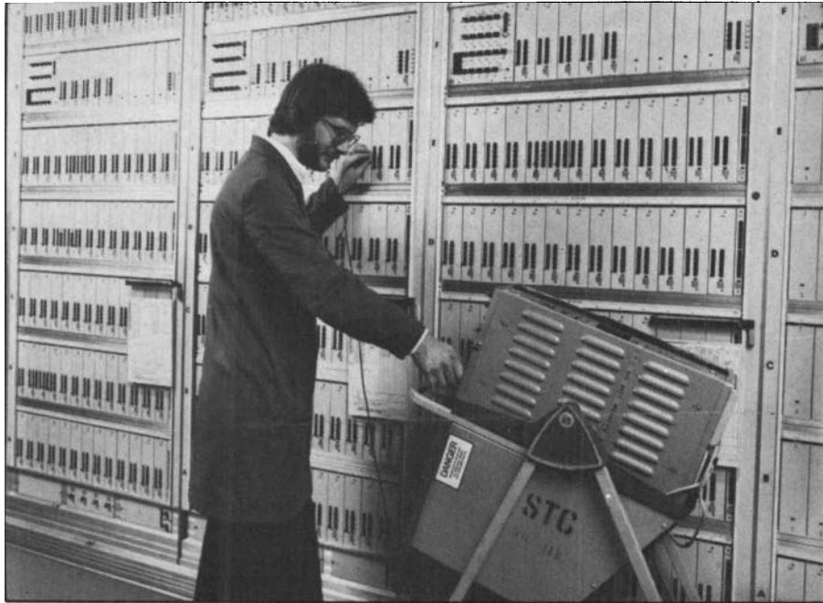
5 Final adjustments being made to rack units in STC's 100th TXE4 telephone exchange at Bromley, Kent
