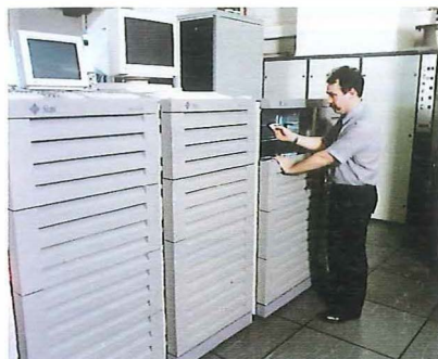
Figure 3—BT WebWorld servers in the Cardiff Stadium House server farm
