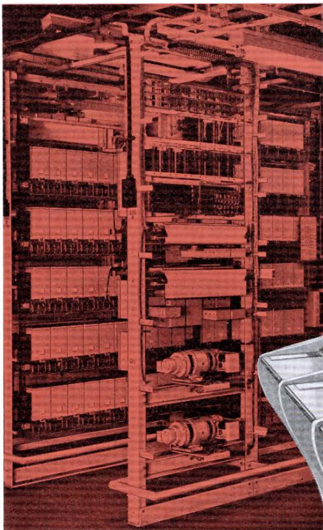
A typical suite of PABX 4 cordless switchboards and automatic equipment racks
