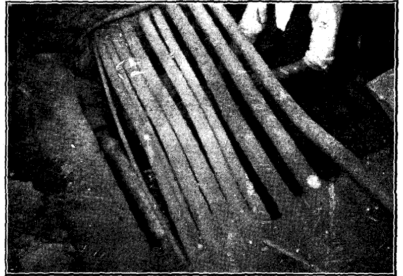
FIG. 1.—Showing Electric Light Cables and Gas Mains, making Work Difficult during the Fitting of Coil at the Split.
