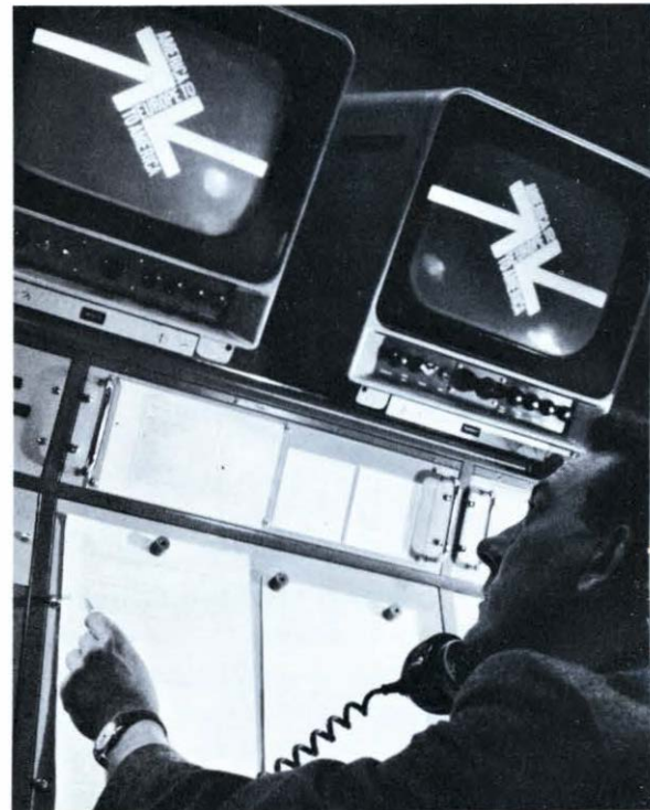
Inside the Goonhilly Downs Earth Station, from which radio signals are beamed to communications satellites. Above: shows monitoring console and, right: the control console during a transmission.
