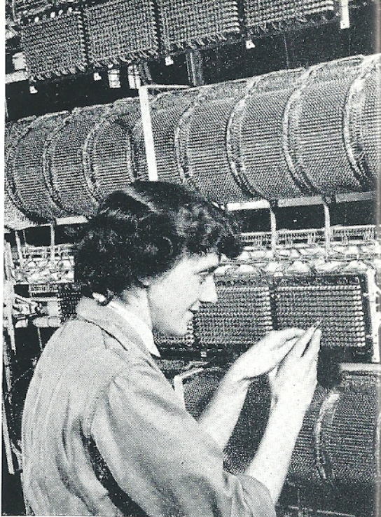
Tag block wiring on motor-driven uniselector rack
