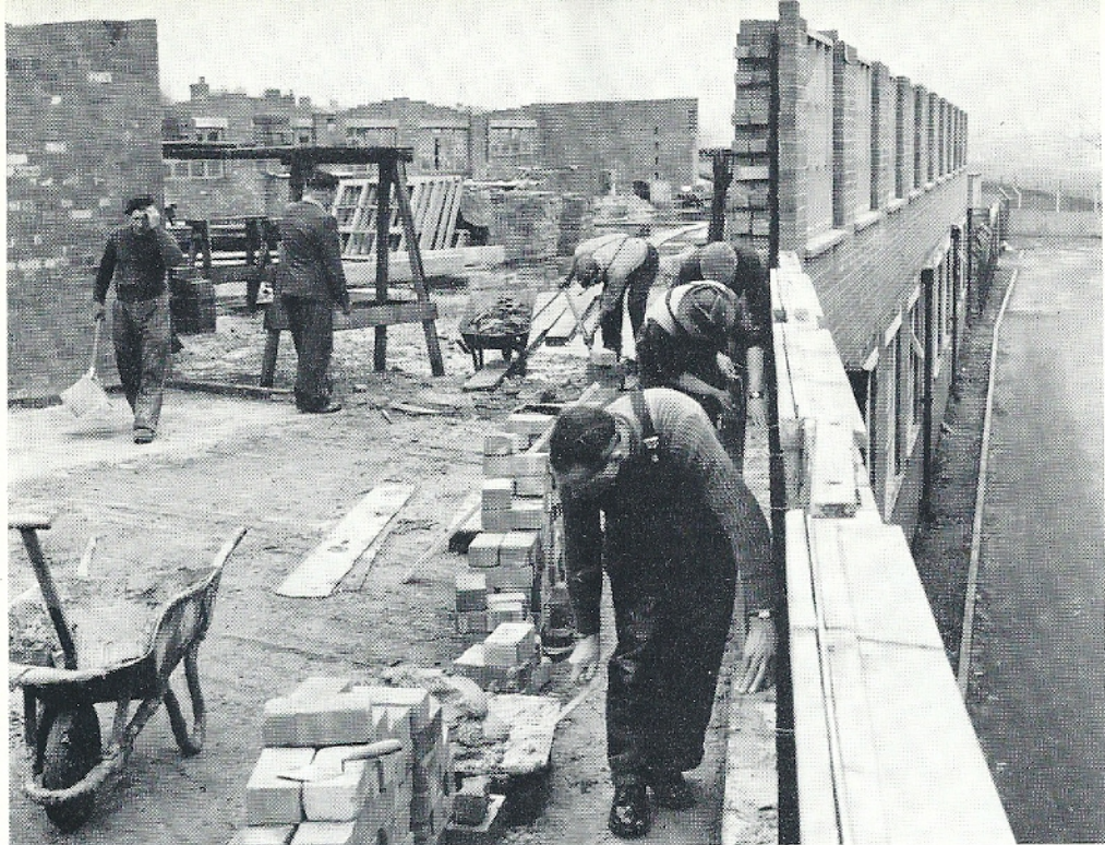
Early work on the construction of new assembly floors at the Wigan factory. A flat-roofed extension, built three years ago, gave the opportunity to construct another storey. The new extension will be completed soon and manufacture will begin in the autumn
