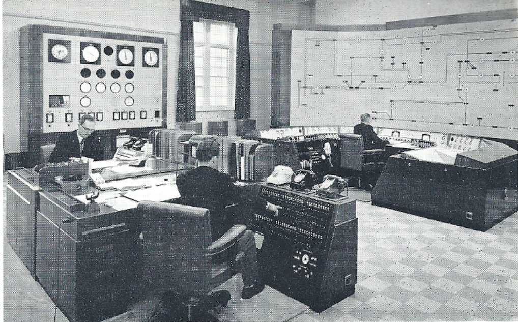
A control room manufactured by ATE recently installed at Bristol
