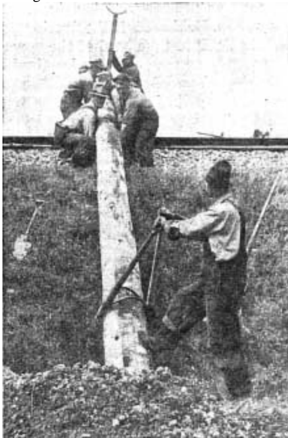
POLE GANGS erect quarter-mile a day, number of poles varying from 26 to 60 per mile
